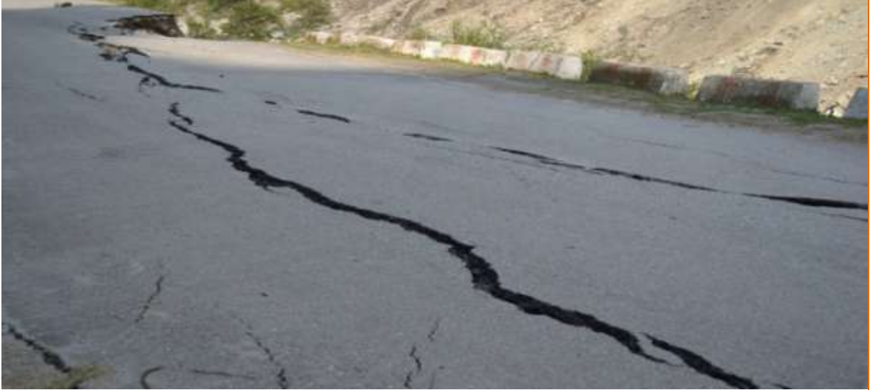
Pic. 41. Damaged road networks
