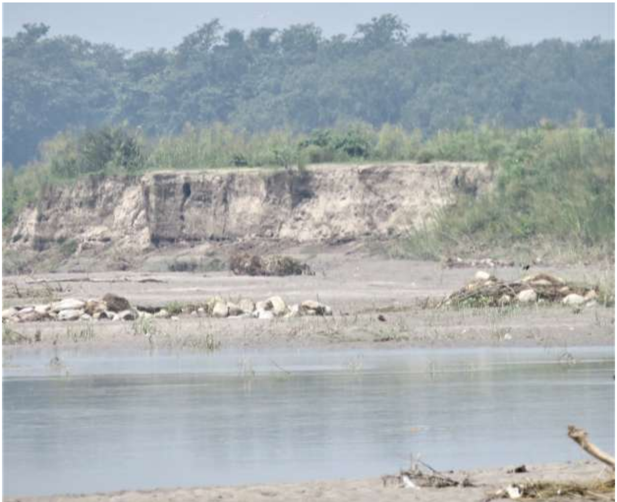
Pic. 172 : Eroded Bank Near Village Damanpuri
